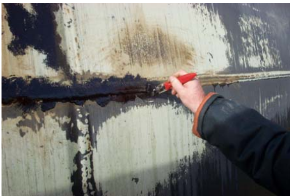
Coating a weld on a poorly prepared saturated surface
