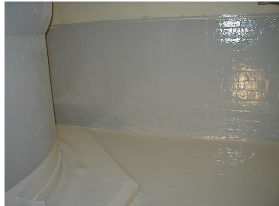
Epo-chem™ RF 500 Bund Lining
