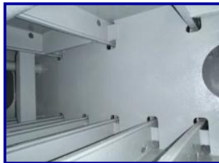
Full surface coated with RS 500P, including all sharp edges, corners and weld areas
